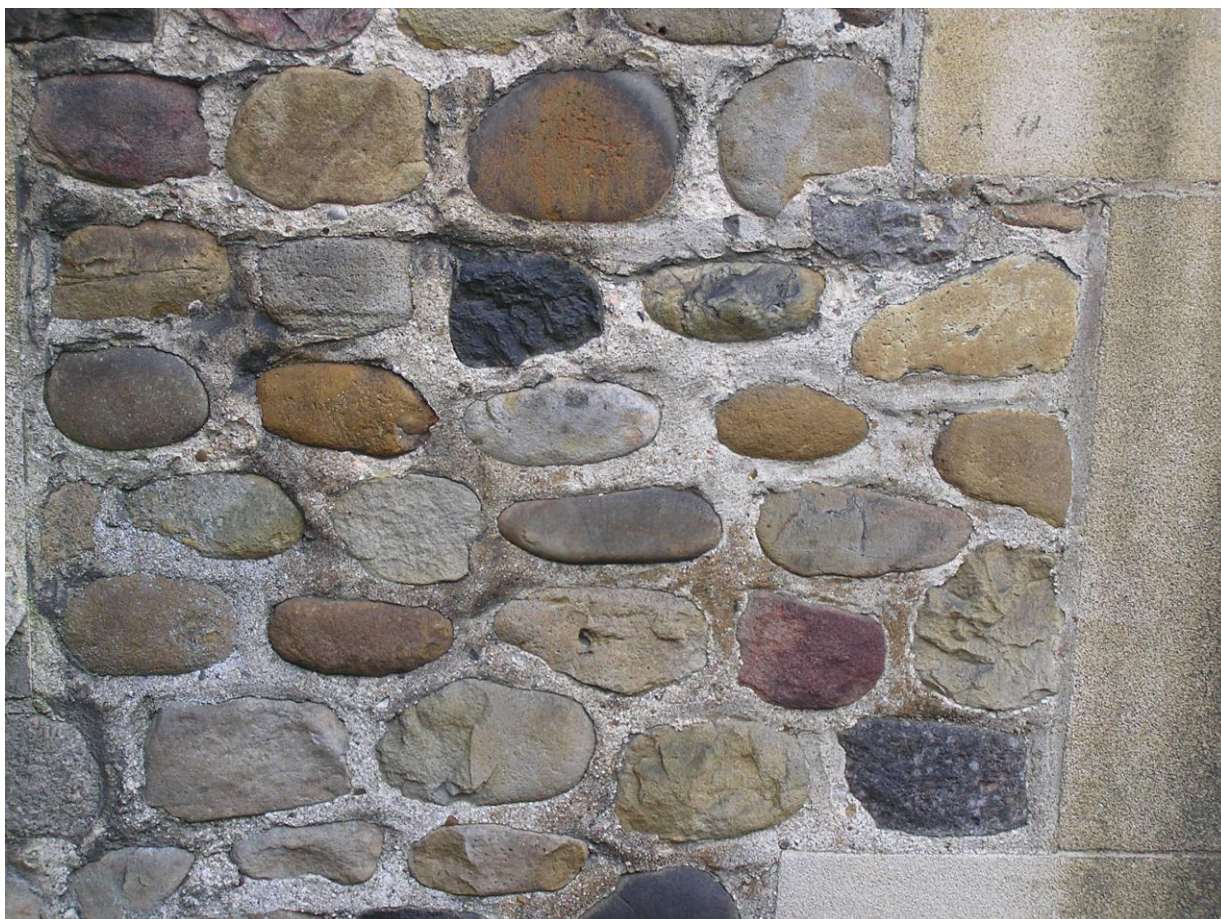
Photo 2. Photograph showing mixed cobbles of red quartzite, together with sandstone, flint, oolitic limestone, granite and gneiss ones, in the entrance wall to Little St Mary’s Church, Cambridge (author’s photograph but facts from Sedgwick Museum Walks booklet),
